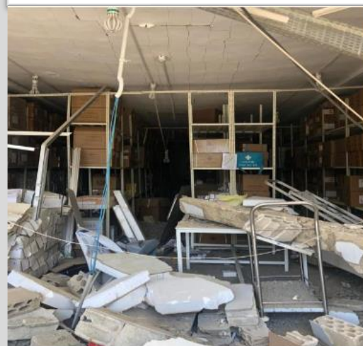
Heavily damaged central drug warehouse, WHO Lebanon
